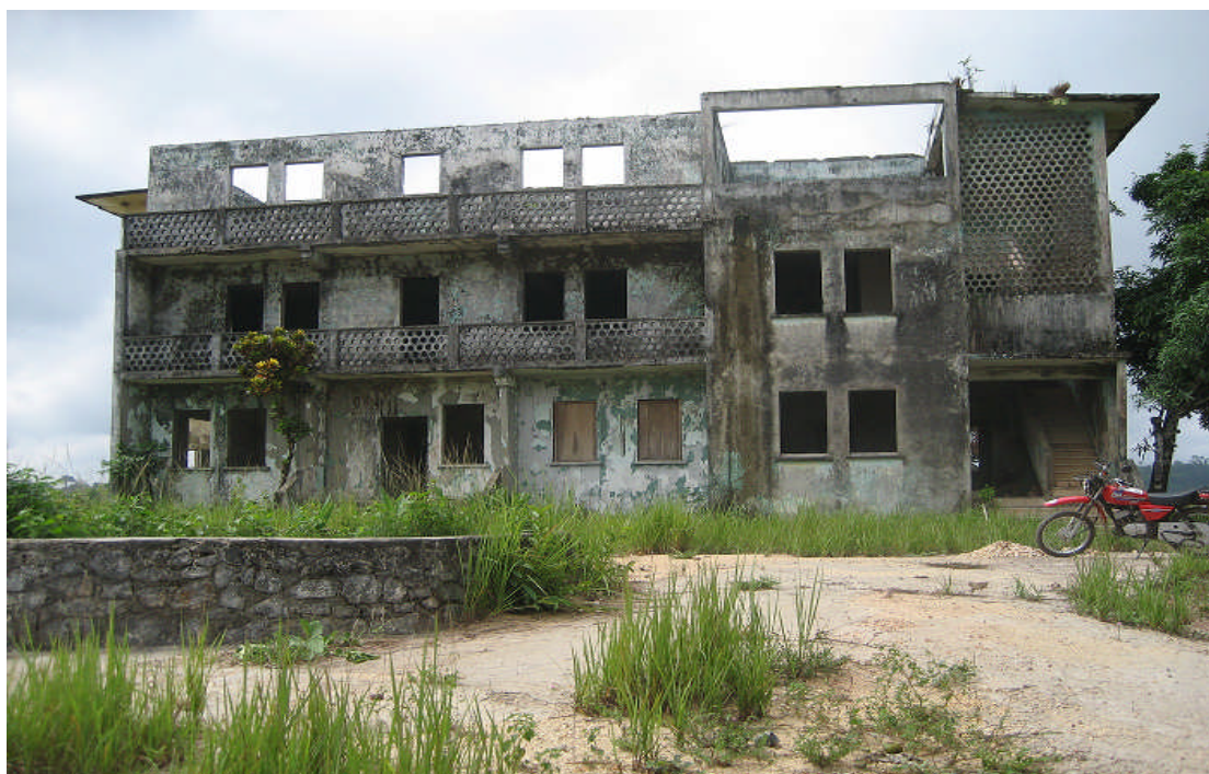
Proposed Development Project in Kolahun: Damaged Administrative Building during the Liberia civil unrest.
